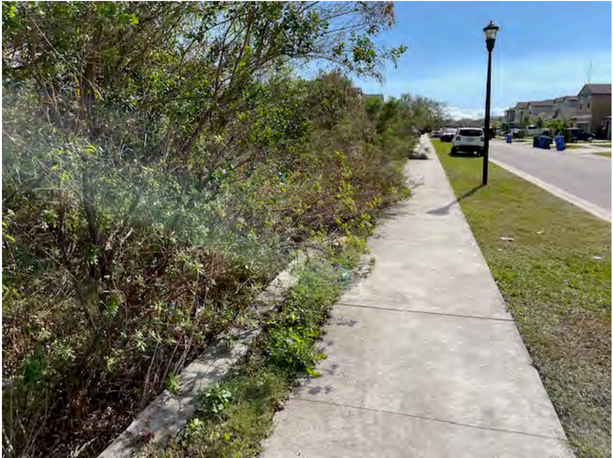
Along Daisy Bloom Pl, the conservation area is encroaching over the retaining wall and sidewalk and needs to be cut back.
