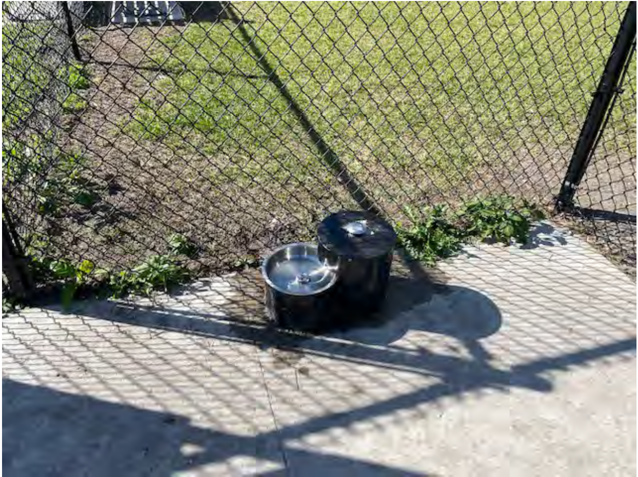
The dog park water fountain is now functioning properly.
