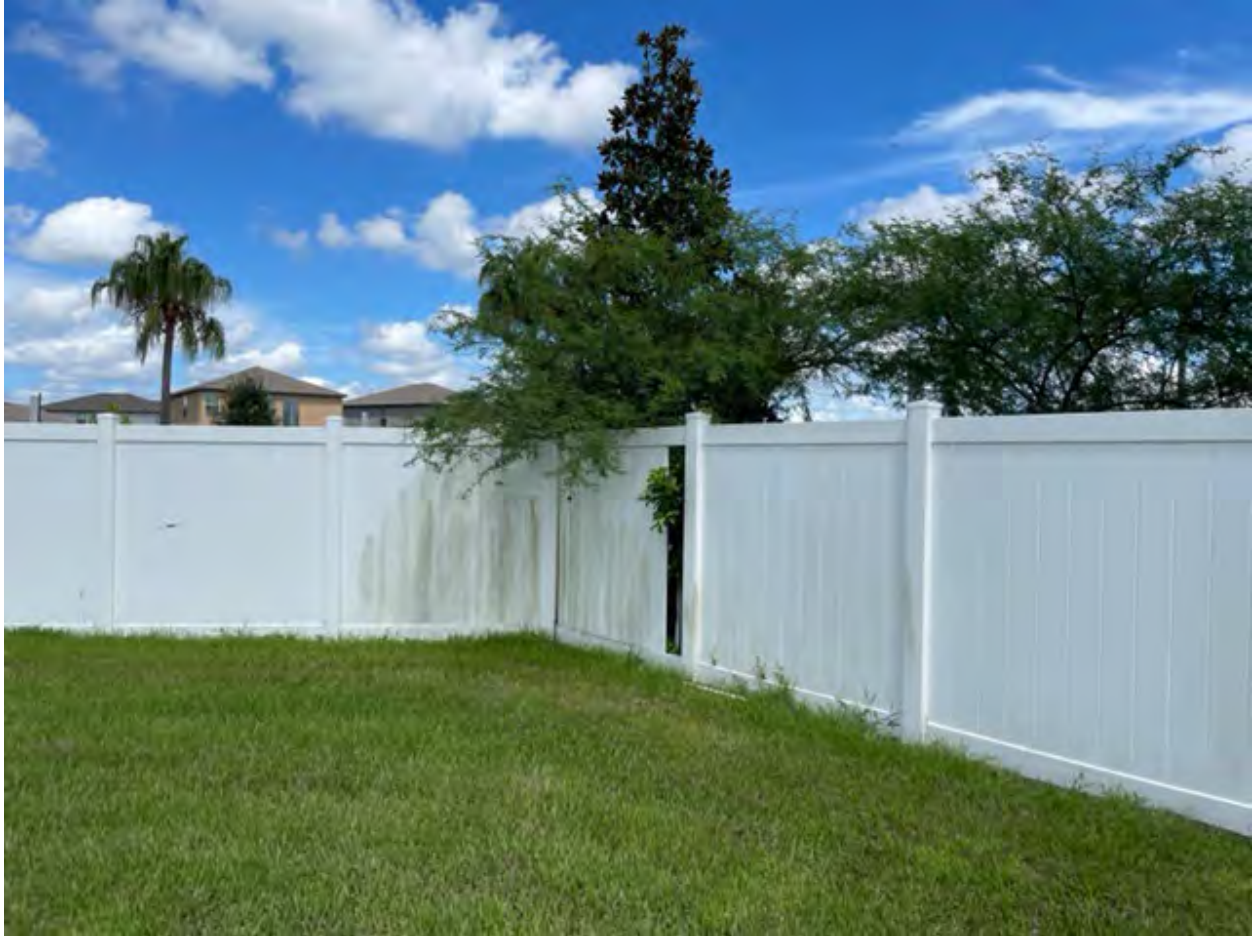
Fence picket is missing behind the main entry, accessible from Ginger Lily Court.
