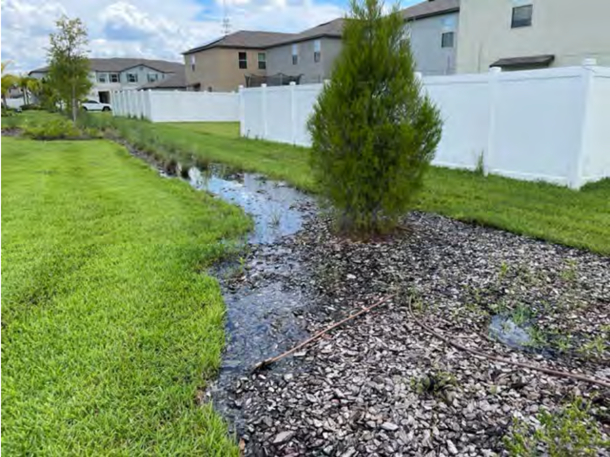
Water pooling up in landscaping bed at the far north pocket park along Samuel Ivy Drive. Looks like an irrigation leak.
