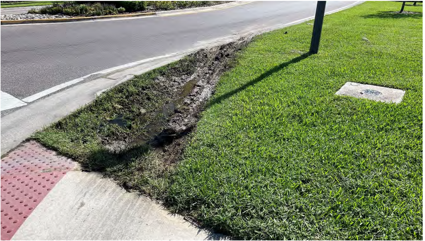
Trucks have been rutting up the turf at the corner of Wild Senna and Camden Fields. We may want to concrete that section.
