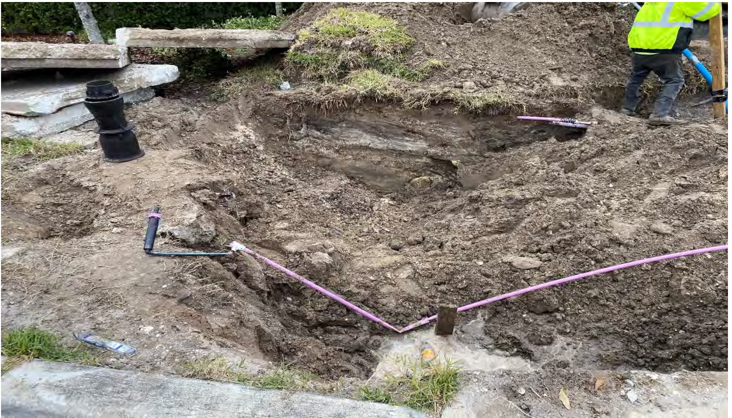
The utility company has torn up the front entrance repairing a water valve. District's irrigation will be repaired by them upon completion.
