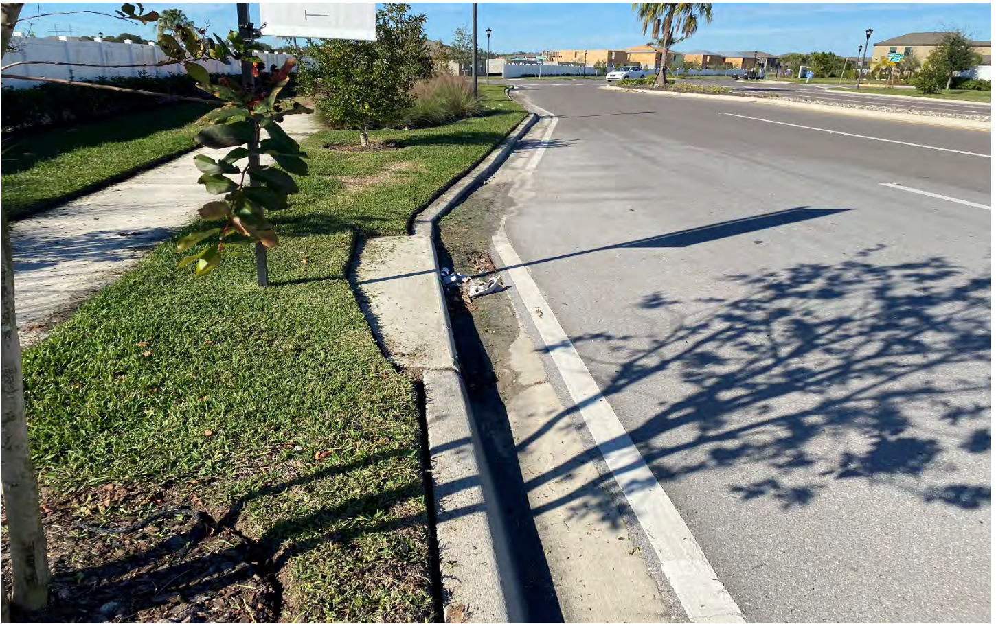
Street gutters need to be cleaned.
