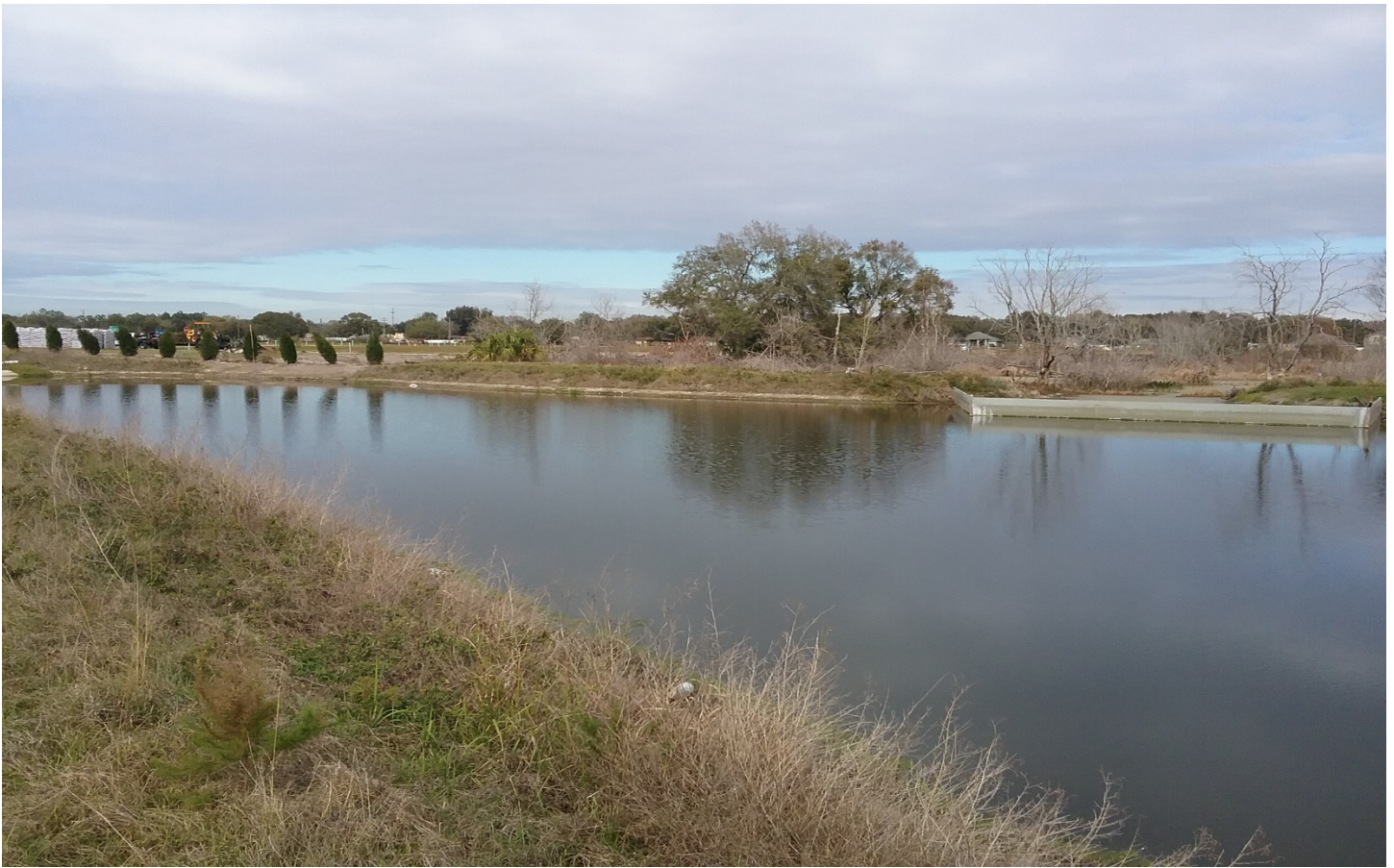
Pond 2 has some trash and the bank needs to be mowed.
