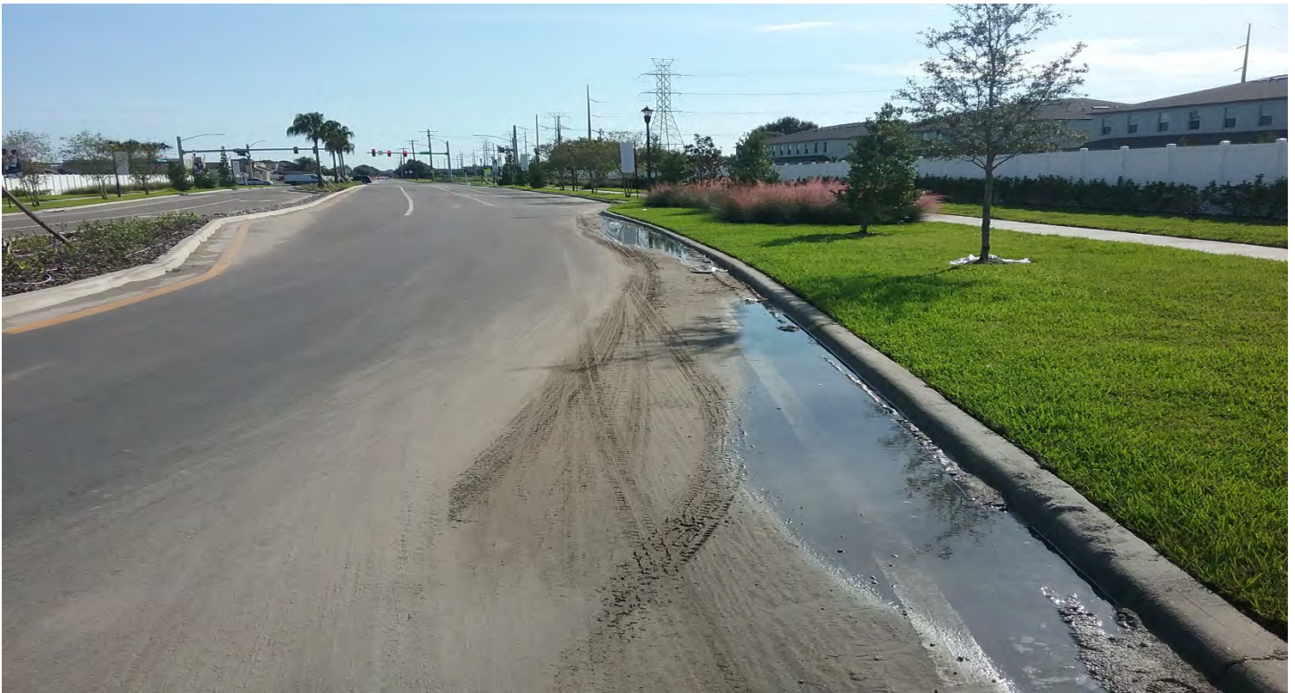
There's a lot of dirt in the curbs along Camden Fields.
