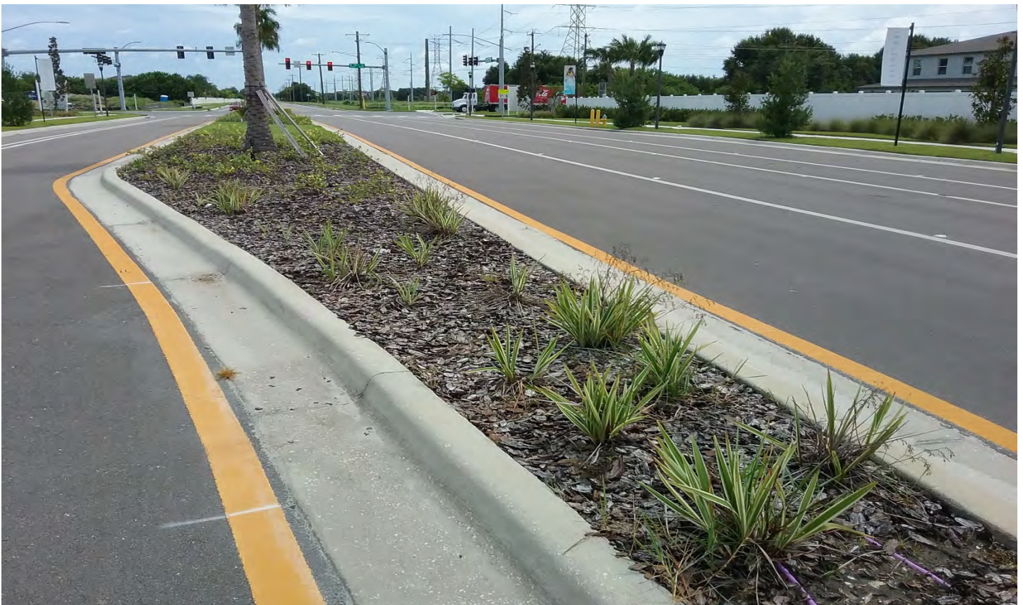
Flax lilies doing poorly due to excessive moisture. The bed should be elevated before replacing the plants.
